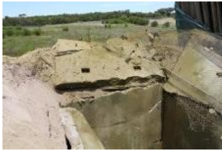
Above: Unsupported parapet walls toppled to sides.
