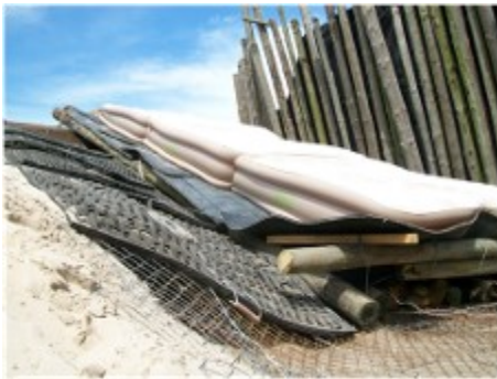
Above: Water mattresses placed on top of gum poles and conveyer belting to resist blast and to form a water barrier during detonation
