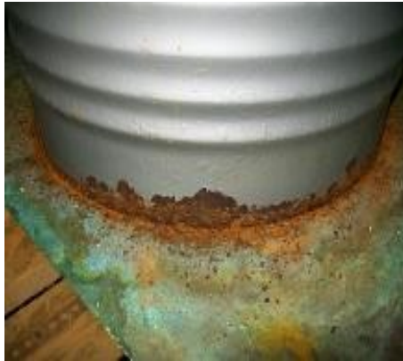
Galvanic corrosion formed between drum and copper plate
