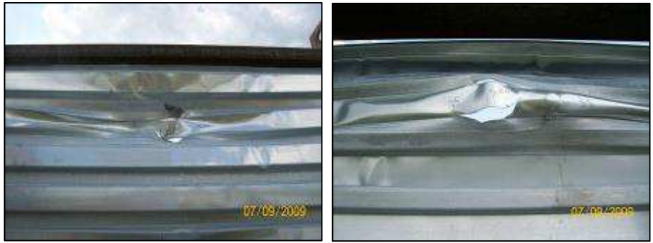
Figure 5: Front and Back of Corrugated Metal Panel (Post-Impact)
