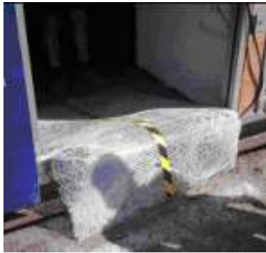
Figure 6. Failure of daylight film application
