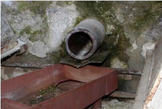
Figure 13 - Drain outlet into building 203
