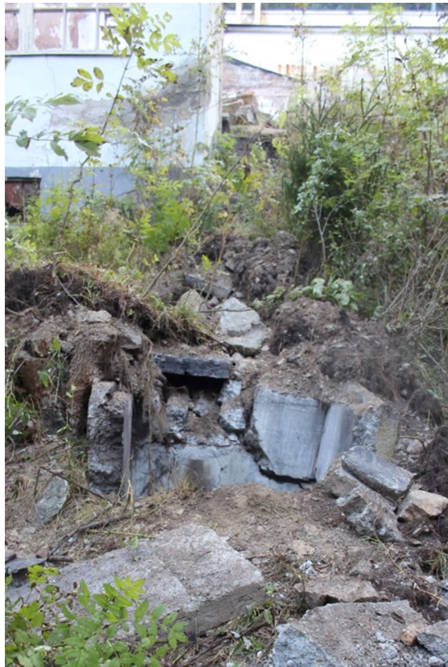
Figure 20 – Line no. 2 with damage by additional explosive
