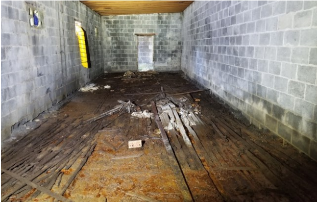
Before - wood on interior walls collapsed and covering 1,300 pounds of sweating dynamite
