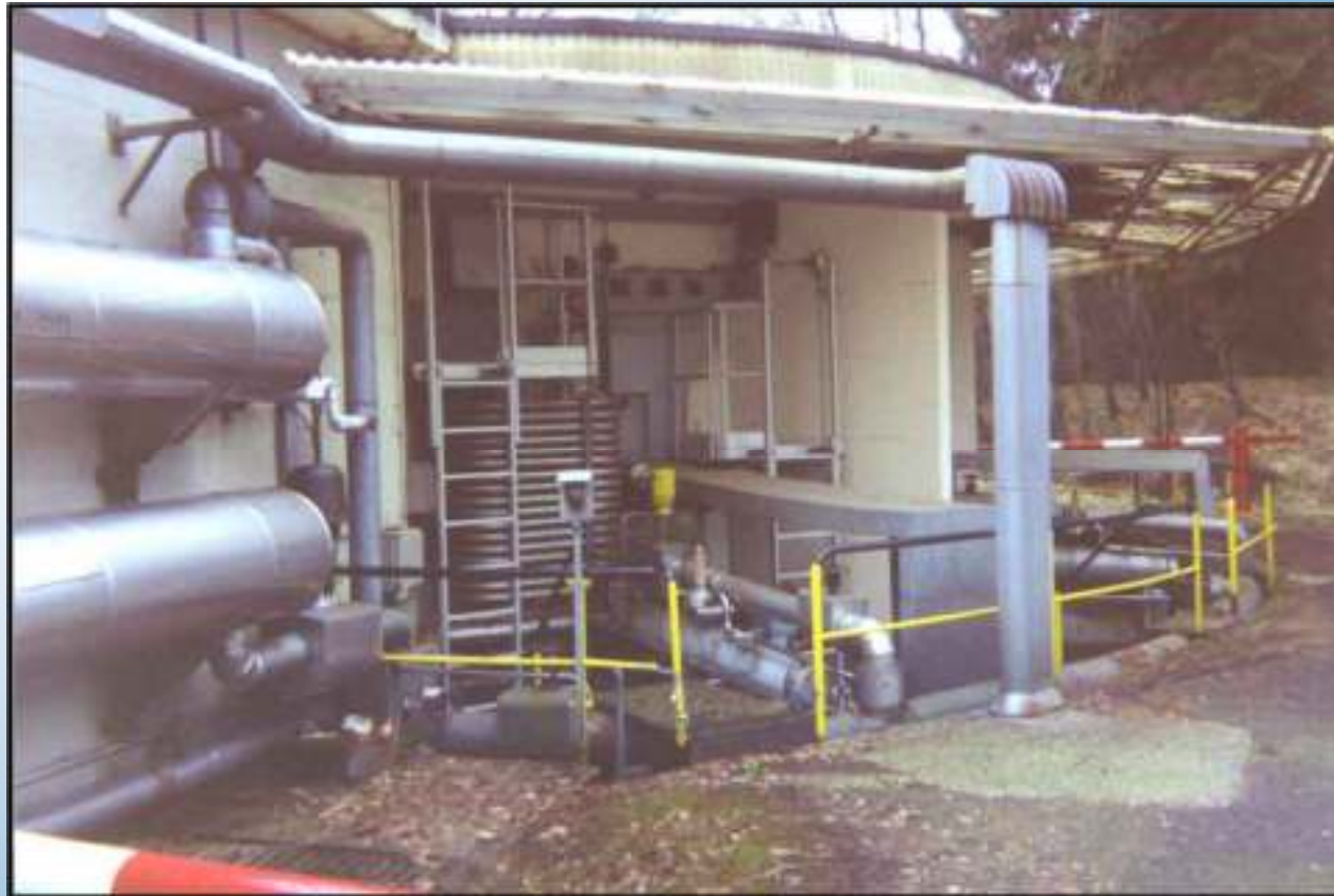
Building 200 (one of two Nitrators & Related Equipment)
