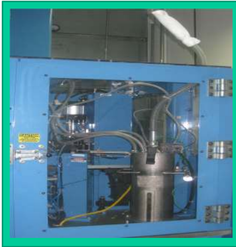
Electrically Continuous Vacuum System
