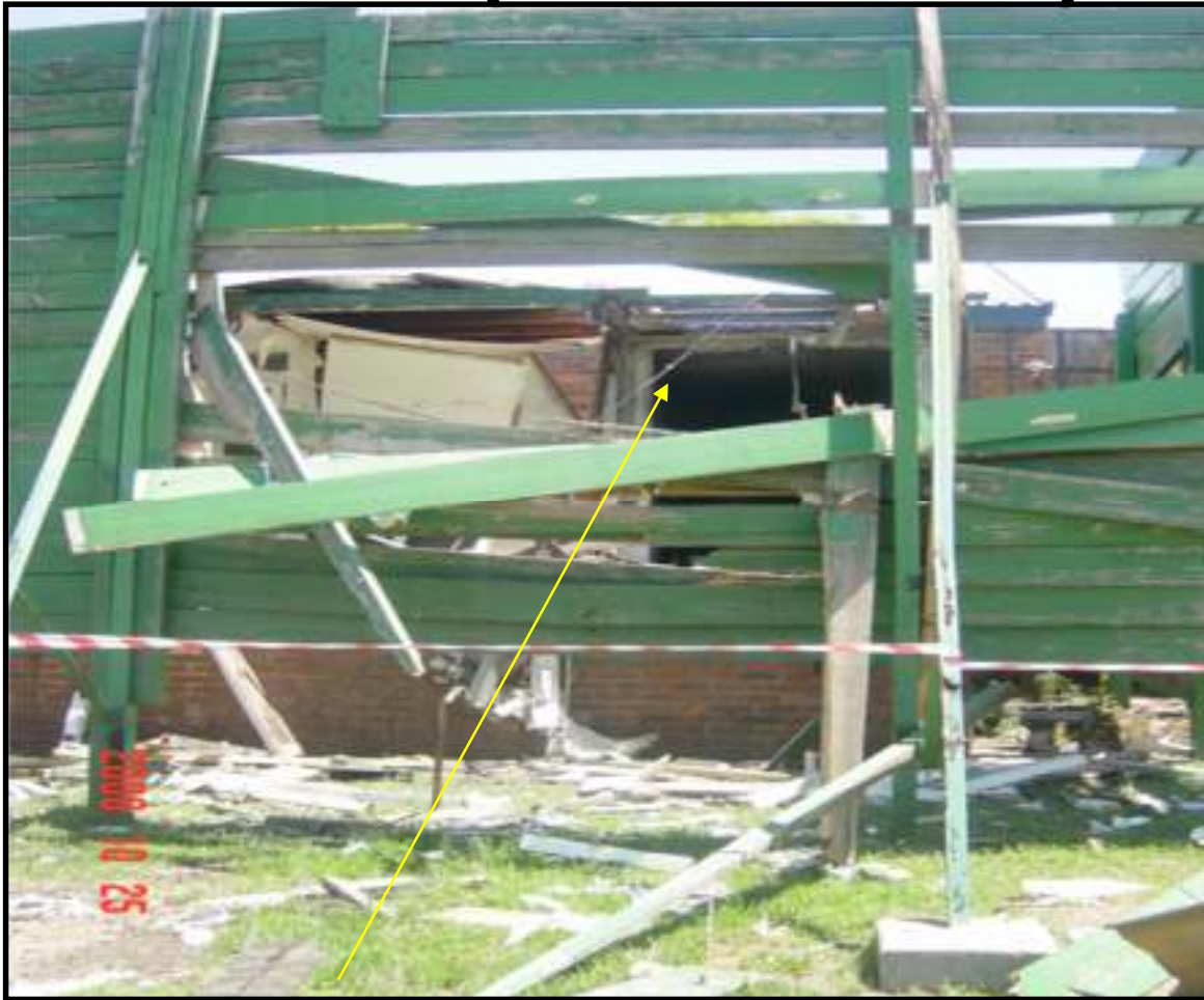
LARGE HOLE CAUSED BY THE EXPLOSION
