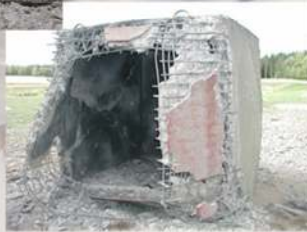
Closed door, Water mitigation (6 l water)
