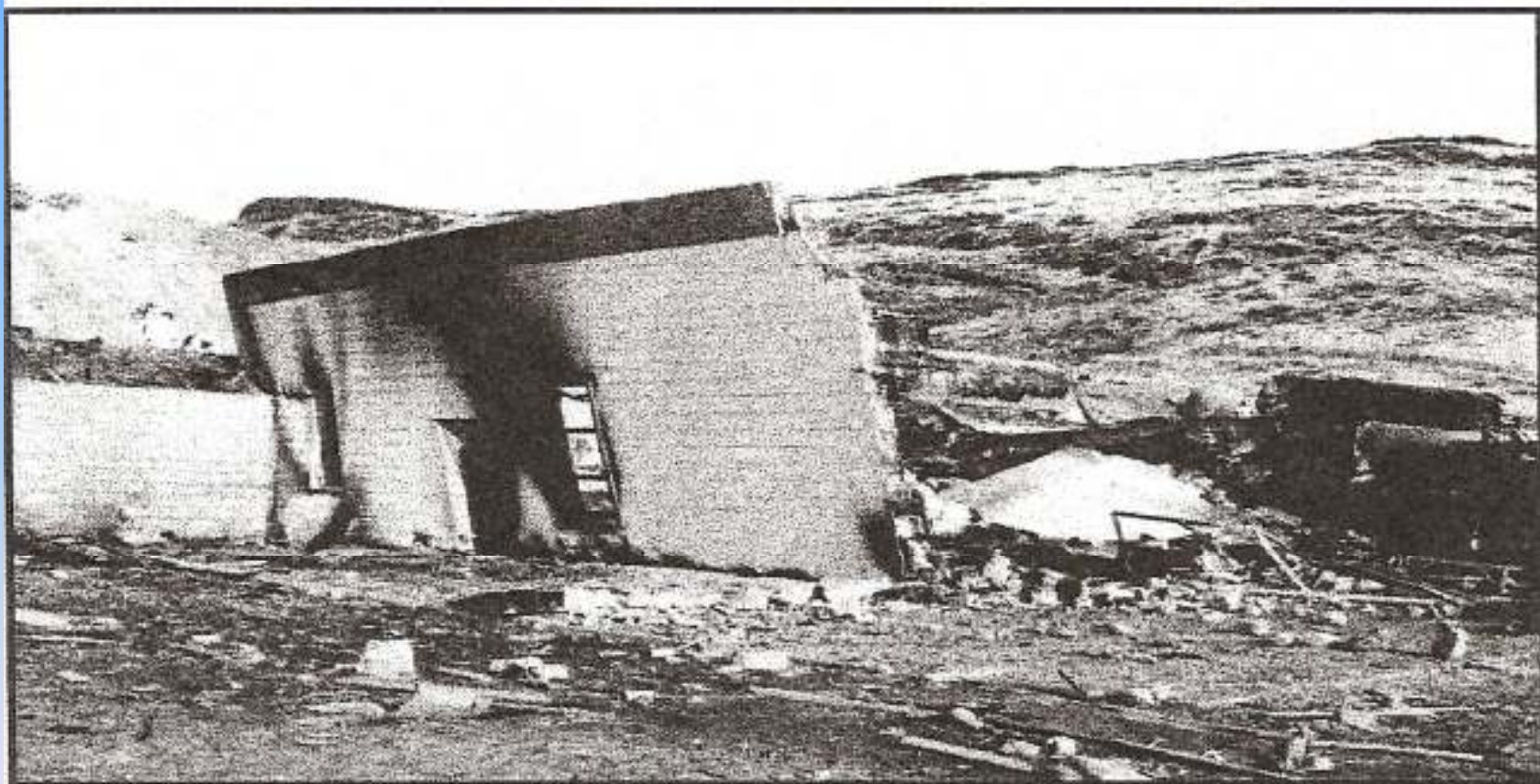
Figure 7. Booster Room 1 After Explosion
