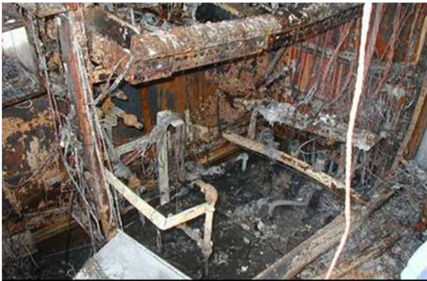
Pneumatic Air regulator which fed the fire after the blast
