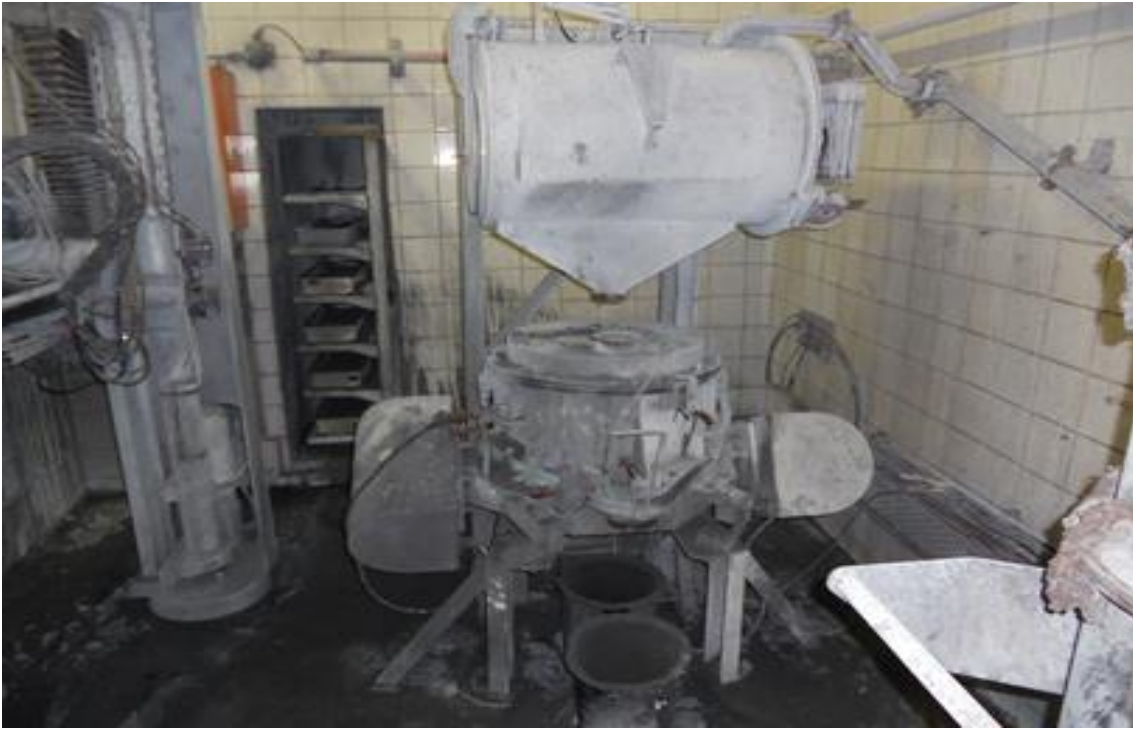
Picture of the damage and equipment.
