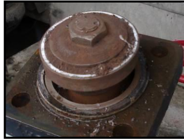
Picture 4: Dismantled gasket showing slag particles that contaminated the Teflon sealing
