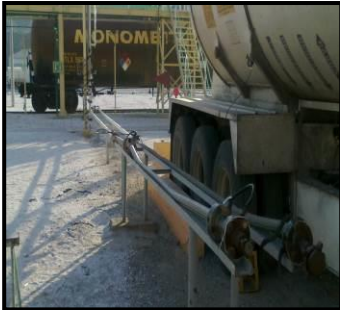
Picture 1: MMA unloading area with tanks and unconnected discharge hoses
