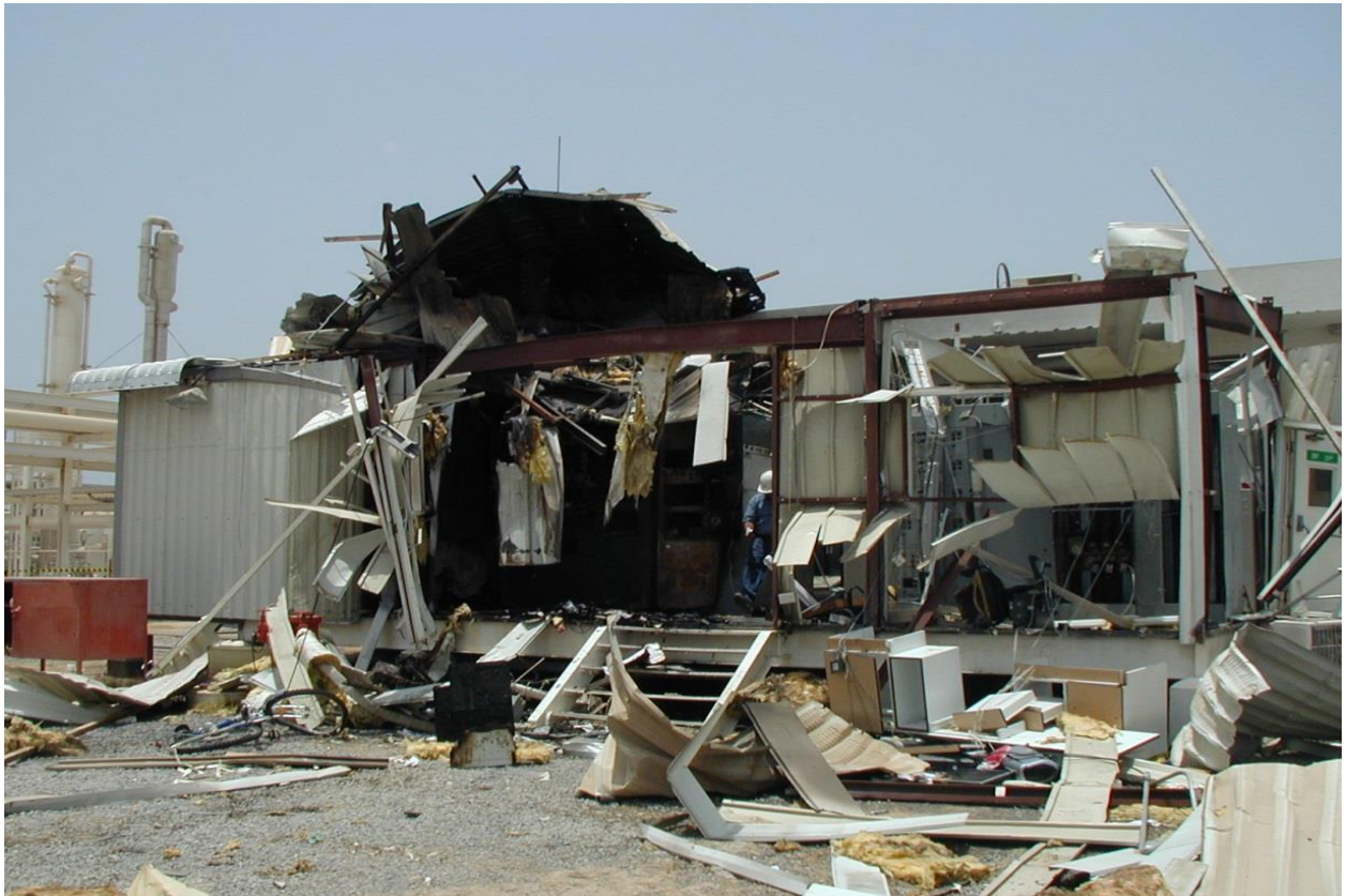
Figure 2: The Central Control Room annex Motor Control Center after the explosion.
