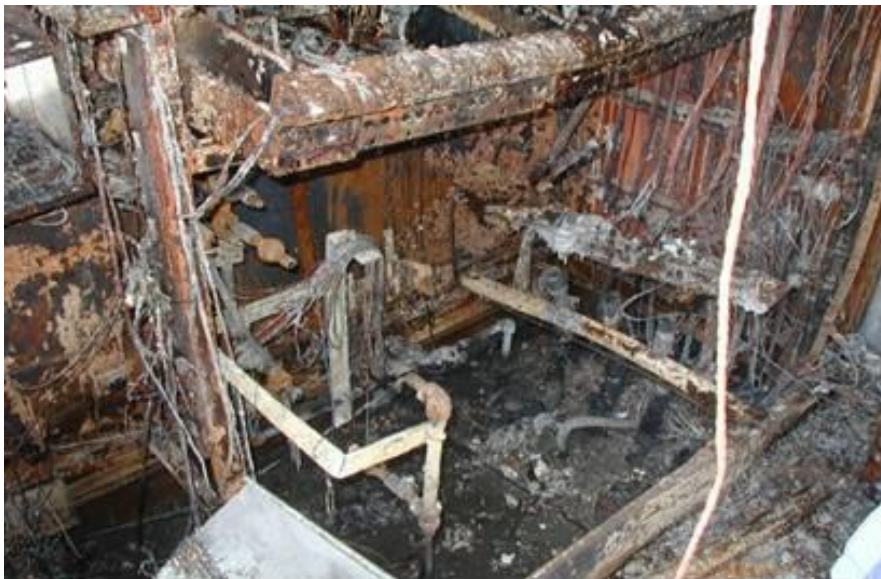
Figure 3: The pneumatic system with regulator after the explosion.
