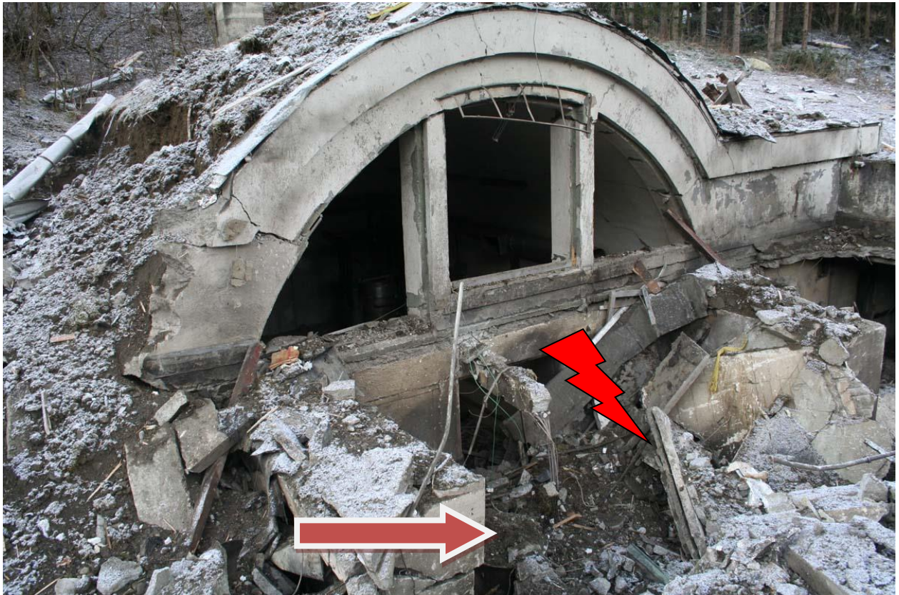
Figure 3 – Buried and trapped mixing bowls with explosives
